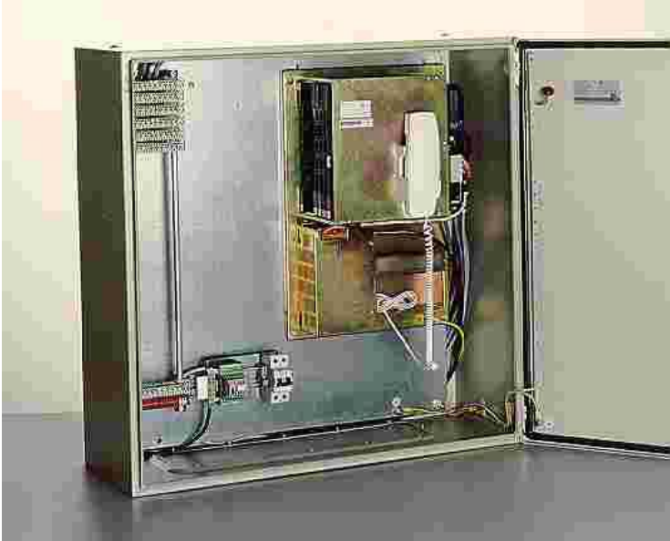
Fig. 1-2 ECS-FD96 in wall mount cabinet
